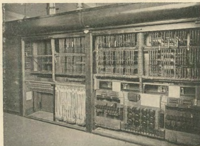
Rear View of Toll, Test and Morse Boards
